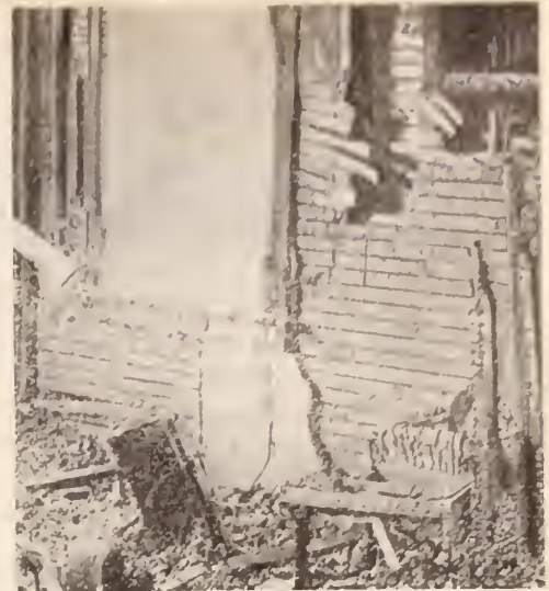
Metal Lath used in place of combustible lath might have saved the life of the woman who was trapped in this fire.
